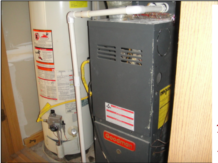
Photo: New Hot Water Heaters and Furnaces
