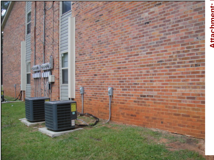
Photo: New Central Air Conditioning Units
