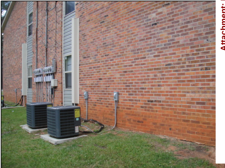
Photo: New Central Air Conditioning Units
