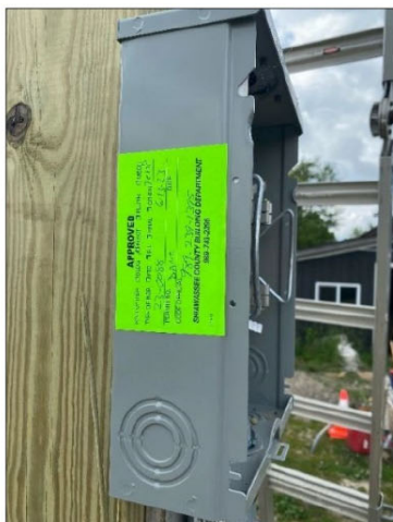
Meter socket inspection sticker.
