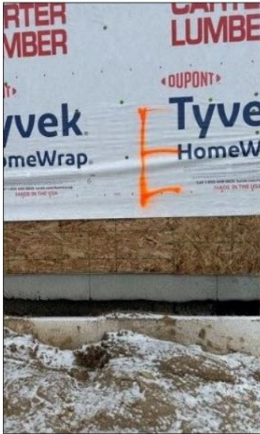
Meter location marked.
