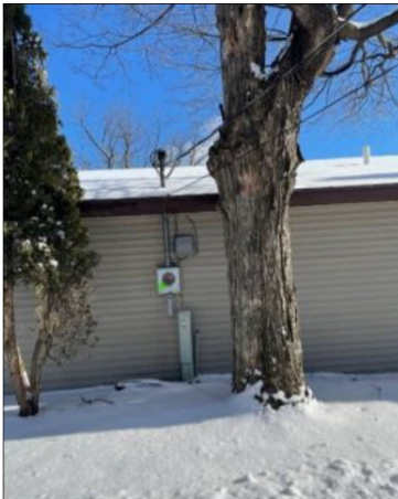
Approved overhead service, meter set only.
